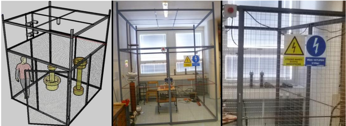
Fig. 1: Design and realization of the high voltage cell.
